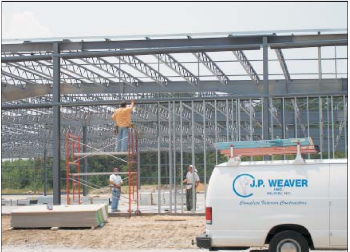
Above, construction workers finish the framing on 47,000 sq. ft. Nashville, NC facility.
